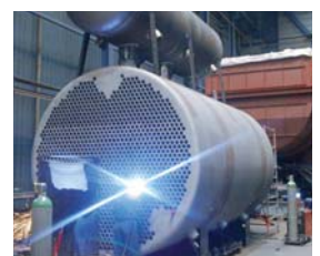
Waste heat boiler
